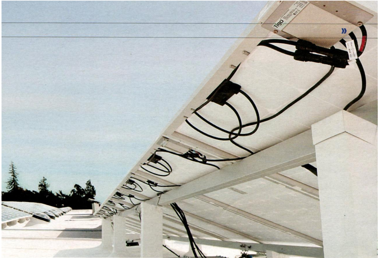
Young but growing: Power optimizers have been on the market for just a few years, but they are already gaining traction among commercial customers. This 780 kW PV array at the headquarters of headset manufacturer Plantronics Inc. in Santa Cruz, California, is equipped with power optimizers from Tigo Energy.
