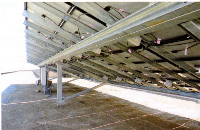
Power optimizers from EIQ Energy were incorporated into this 1.2 MW plant at Granite Construction in Coalinga, California. The installation uses thin-film modules from Solar Frontier.
